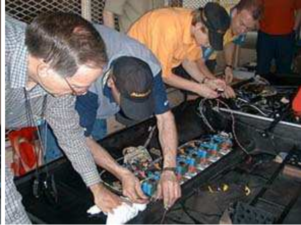
The team work hard cleaning the electrical array
