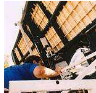
Day 4, Andrew replaces the damaged solar trackers (click for a larger image)
